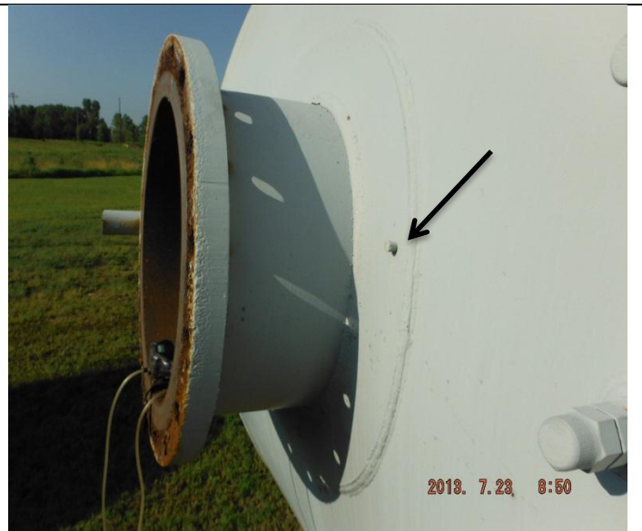
Repad plugged with threaded plug
