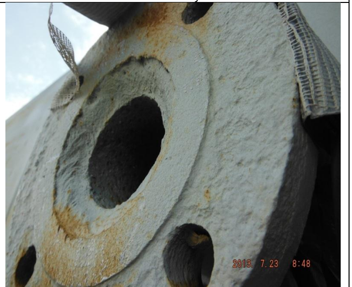
Corroded Flange Face
