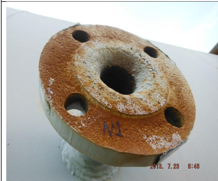
Corroded Flange Face
